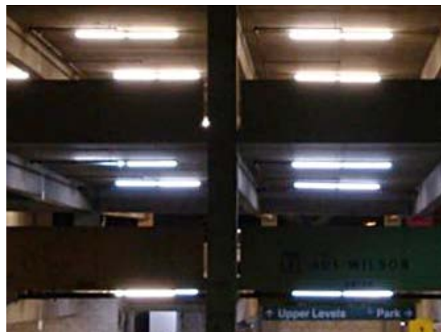
First CECIP project. Photo taken during mid-project tests showing the new LED lighting on the second floor of the parking structure compared to the old T8 fluorescents on the third floor.
